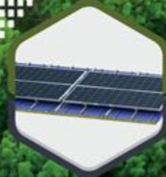
Solar Kepli Panel
